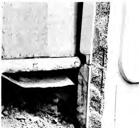
Photo 16. This is a detail of photo 15. Drilled expansion bolts from floor slab (shown) to tilt-up walls failed to hold panel in place. Similar failures occurred where the 3-inch dowels from the tilt-up wall to the pilaster proved to be completely inadequate. E. G. Zacher photo.
